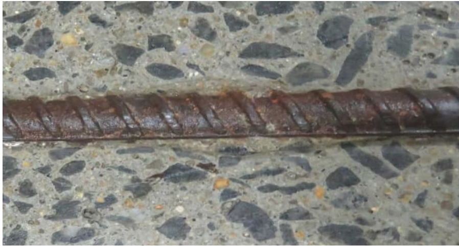
Figure 11. Uniform corrosion due to carbonation.
