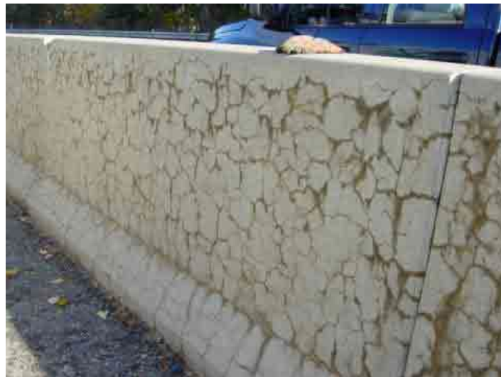
Figure 26: ASR in a concrete structure, with visible map cracking and leaking gel on the surface.
