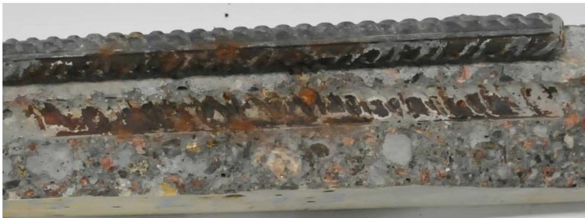
Figure 13: Pitting corrosion in an embedded rebar.
